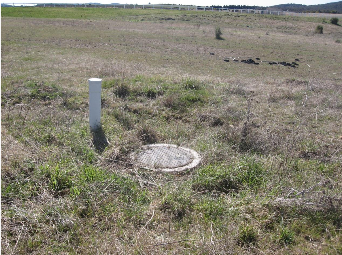
Sewerage Manhole and Service Riser
